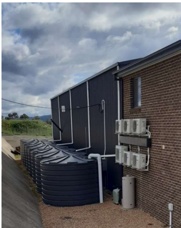
Figure 8 – Campbells Transport Bathurst - Rainwater Tanks
