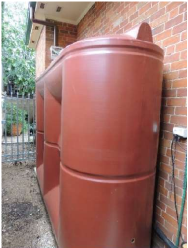
Figure 5 – 5000L rainwater tank
