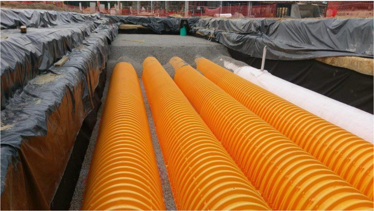
Figure 7 Underground pipeline water storage system 31
